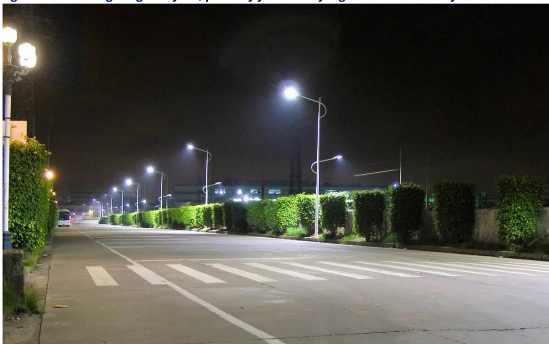
Figure 13. Street lighting in Atyrau, partially financed by a green loan issued by the EDB
